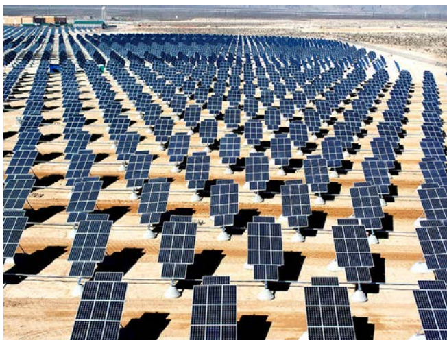
Figure 2: The largest photovoltaic plant to date in North America at Nellis Air Force Base. Attribution: Wikimedia Commons
